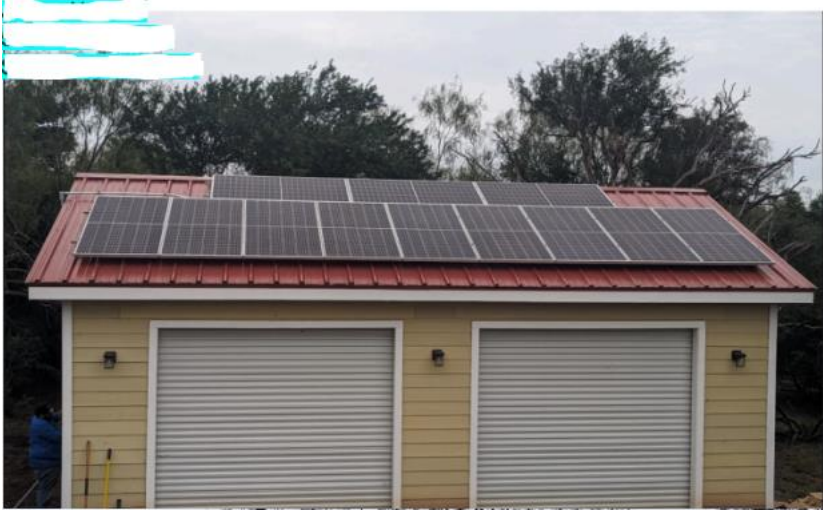
Photo clearly displaying panels installed
