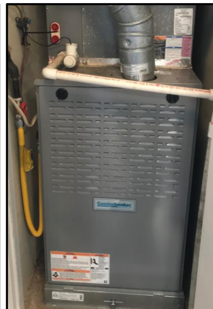
Indoor unit (gas)
