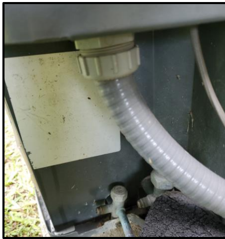
Outdoor unit nameplate unreadable
