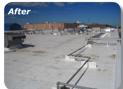
The new roof saves energy and money by preventing heat absorption into the building and minimizing roof temperature.
